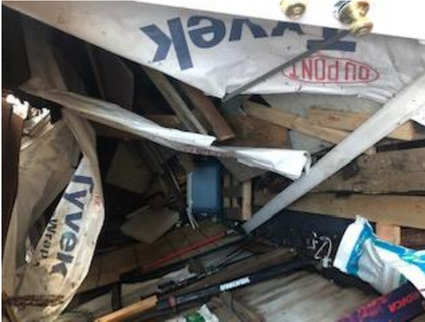
Inside of Garage showing roof collapse
