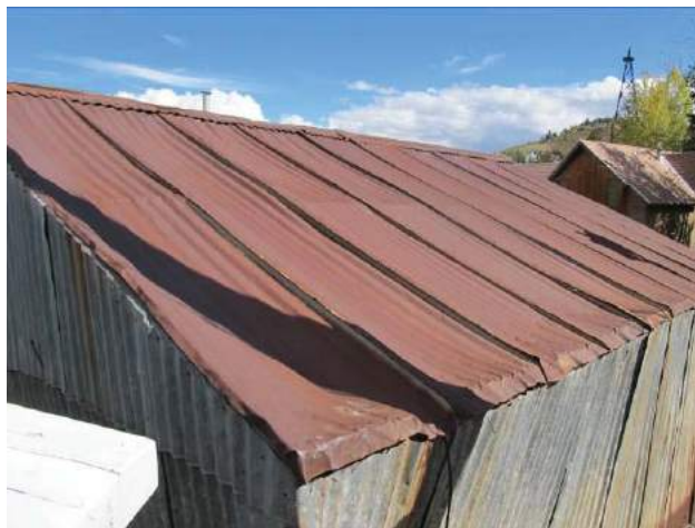
This image shows how the garage is settling in different directions.
