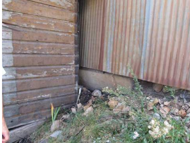
The wall on the left is the original wall between the house and sleeping porch. Note how the garage is pulling away from the wall of the house.
